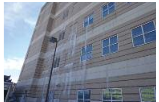
Water freezing as it poured out from the building.
